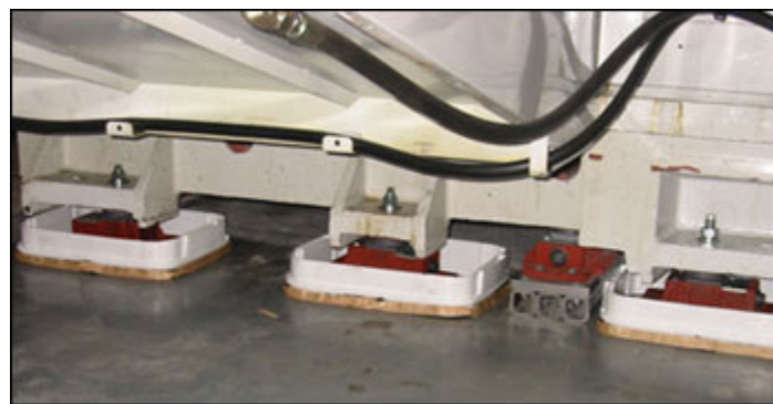
Preparation for the use of epoxy to anchor the machine to the floor. Photo courtesy EOS
